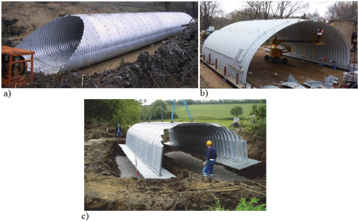
Figure 2.4: Assembly of CSP: a) closed profile on the ground, b) open profile on the RC strip footings, c) open profile on the CSP [36]
