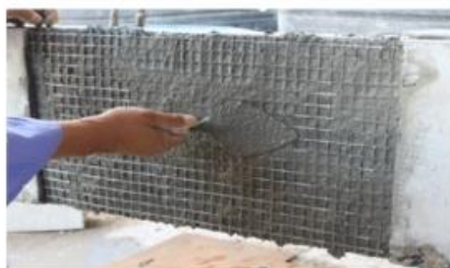
(c) Installation and full impregnation of first layer of fabric (continuous configuration).
