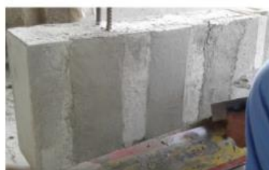
(d) Final layer of mortar and finishing of the surface (discontinuous configuration).
