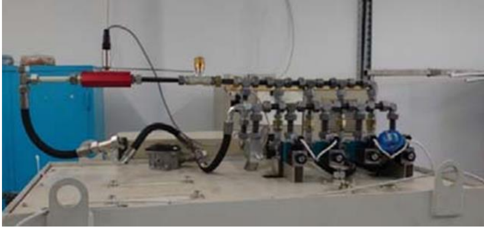
Figure 31. Valves and connection block.
